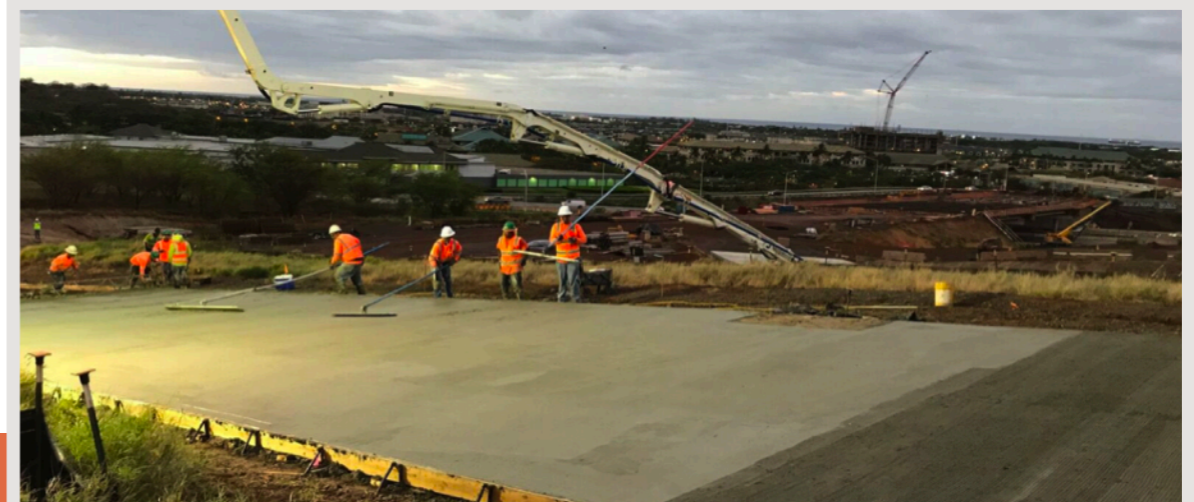
Concrete utilizing CarbonCure's technology from Island Ready Mix being installed at Kapolei Interchange Phase 2.
