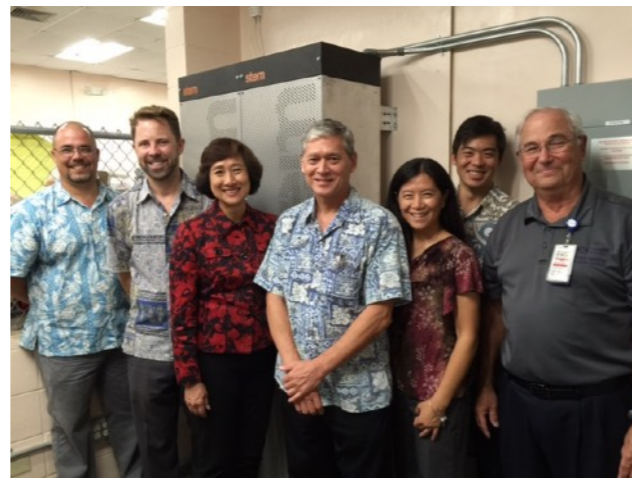
Stem announces its first behind-the-meter storage project with Hawaiian Electric, co-funded by Elemental in 2014
